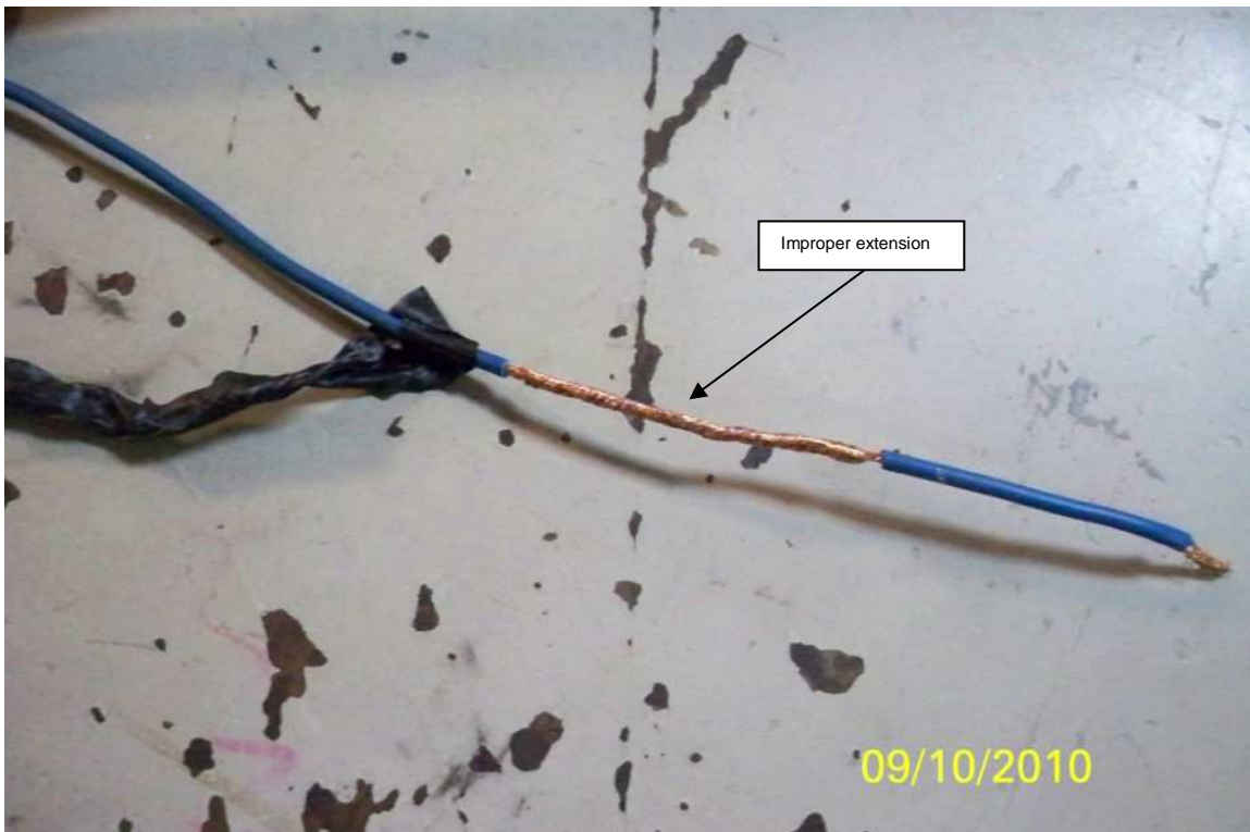
Electric cable with an improper extension of wire
