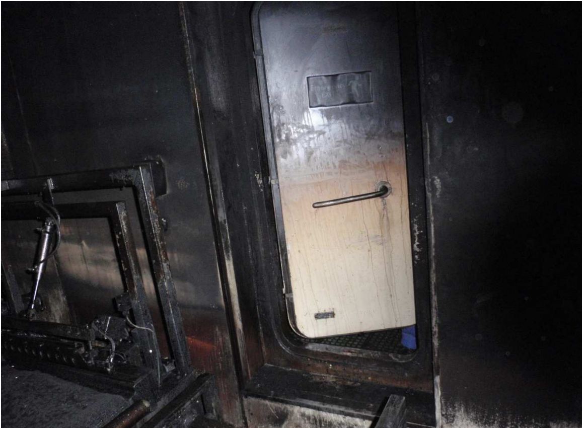
Port side door in bulkhead between processing area and packing room on the 2nd deck (open during fire) Photo: The Investigation Board
