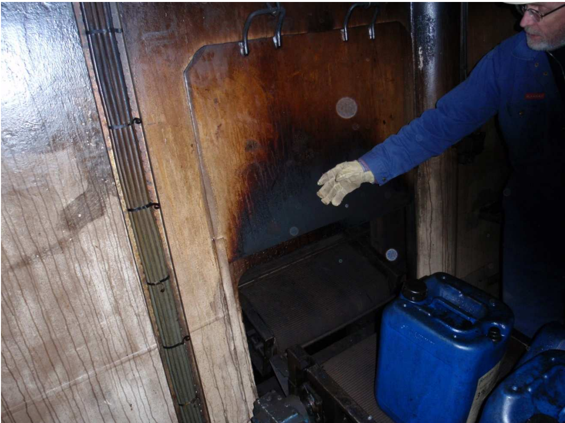
Open sliding hatch viewed from the processing area
