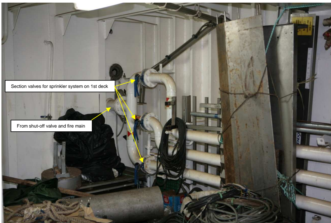
Sprinkler system's section valves for sprinkler on the 1st deck
