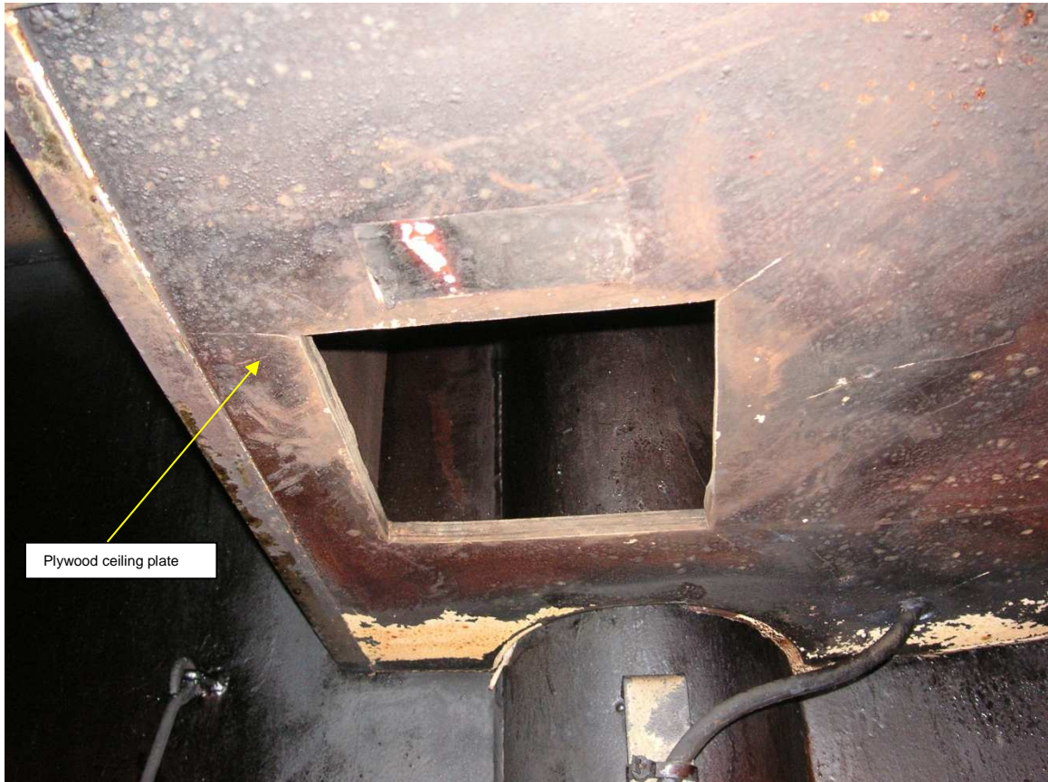
Ceiling plate and opening for operation of section valve for sprinkler system in packing room on the 2 nd deck
