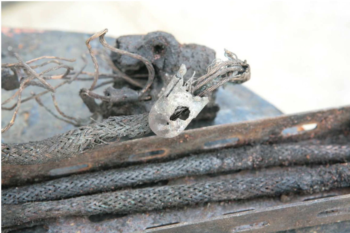
Damage to cable metal braid and cable identification marking caused by arcing
