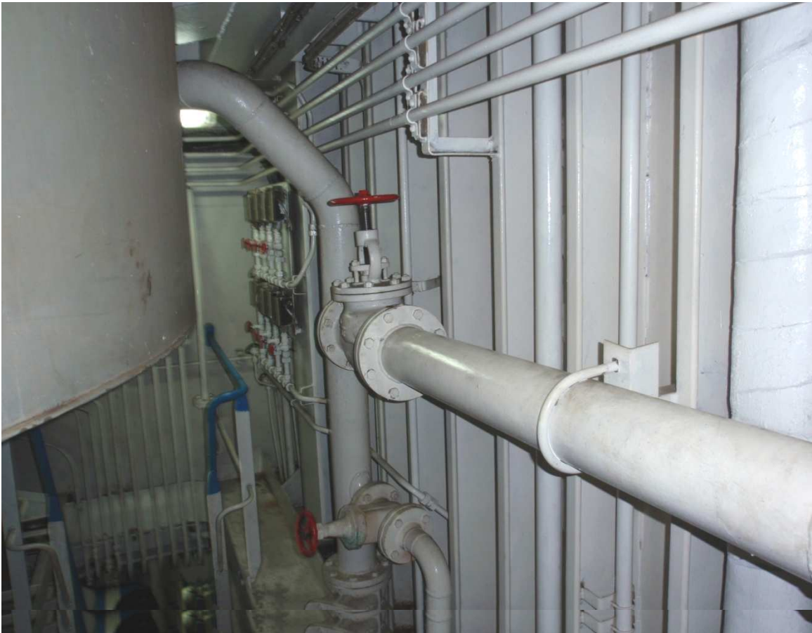
Sprinkler system's shut-off and isolating valve for sprinkler sections on the 1st deck
