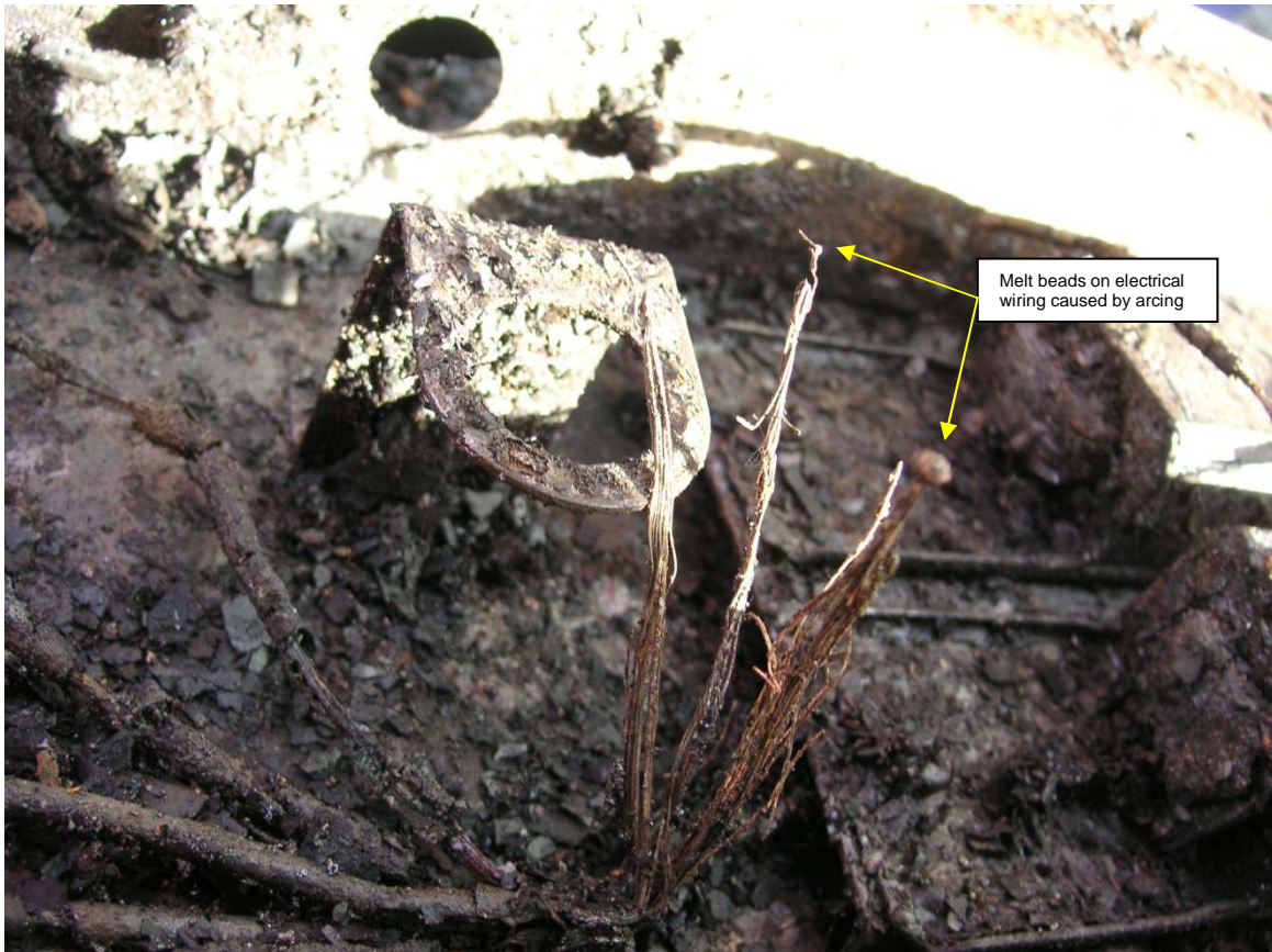
Melt beads on wiring in fluorescent tube fixture caused by arcing
