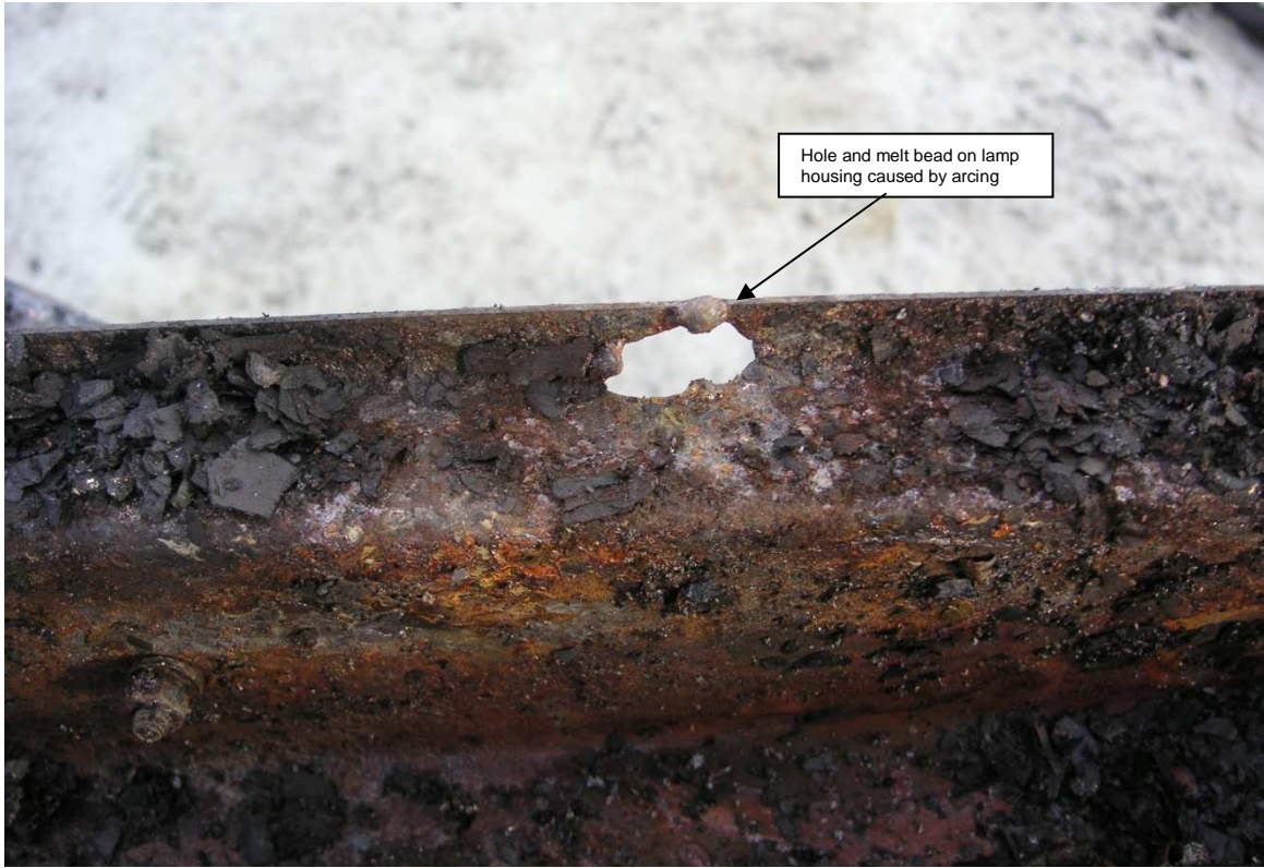
Damage to housing for fluorescent lamp fitting, caused by electric arcing
